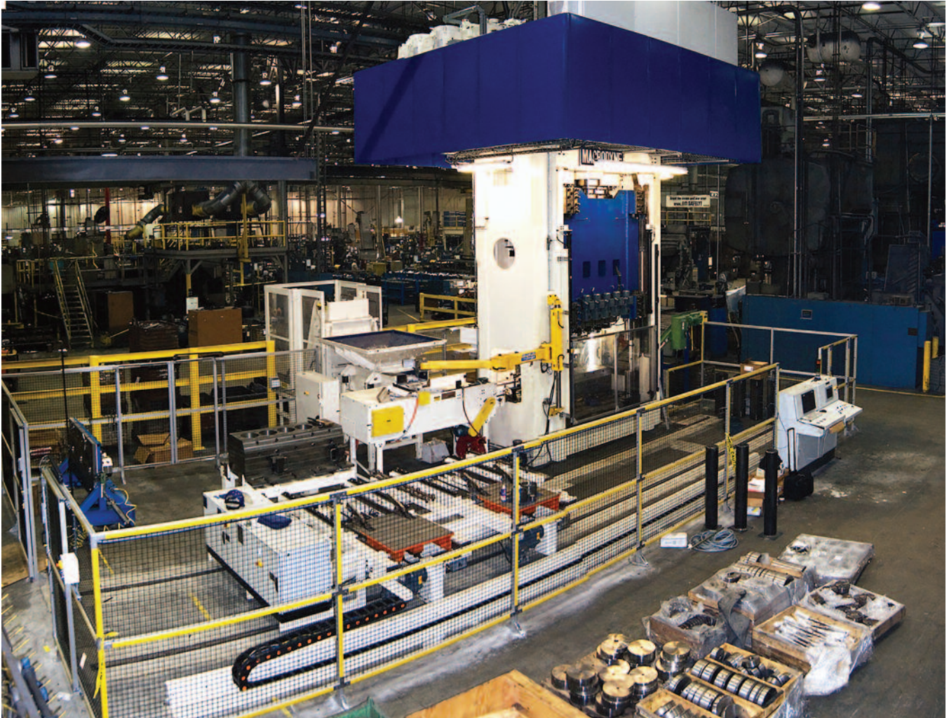
2000 ton cold forming press line
