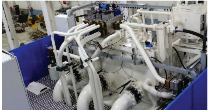
Hydraulic system for a 1000 ton hot stamping press featuring non-welded piping
